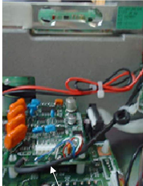
Load cell communication harness
