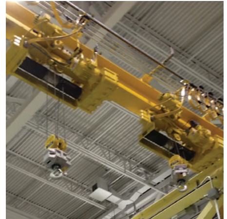
Bridge cranes pair well with a variety of MSI scales, though environment can impact the choice.
