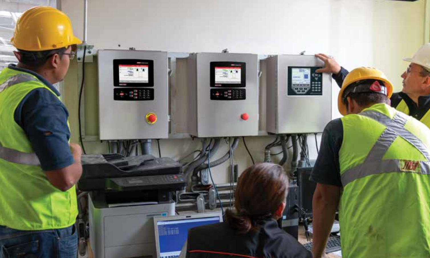
1280 programmable indicators automate the grey and white mortar processes while the 920i controls the bagging line.
