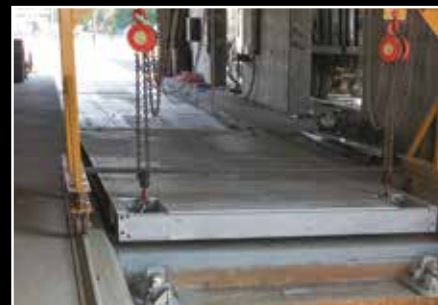
A gantry system enables the entire scale deck to be moved for routine foundation cleaning.
