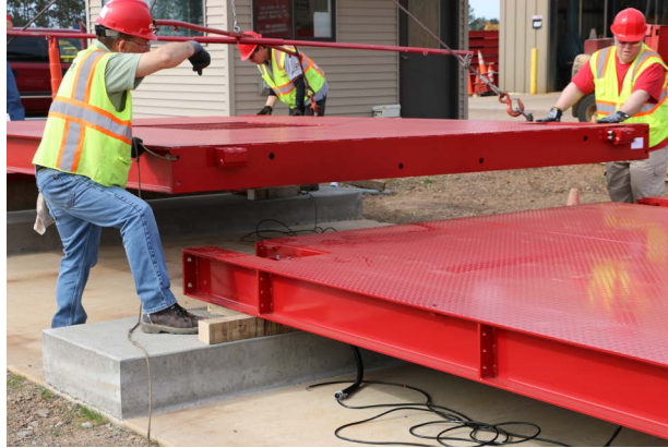
Figure 3-5. Module B Installation
